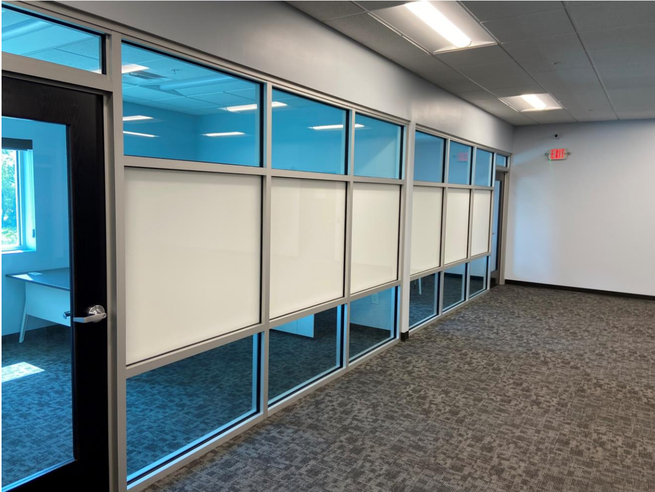
Office area – Doors and bottom panels must be safety glazing Decorative used for writing surface
